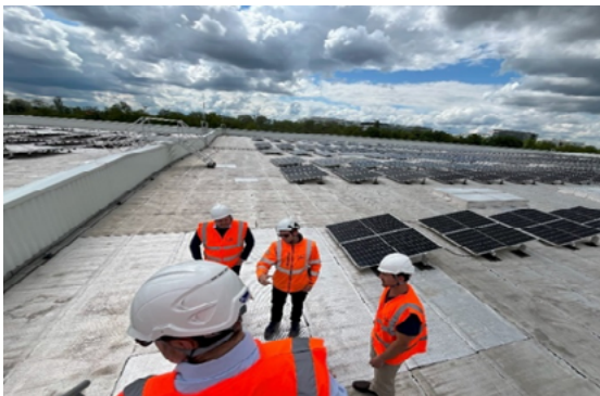
Frontier visited a C&I rooftop solar facility in Val-de-Marne on the outskirts of Paris
